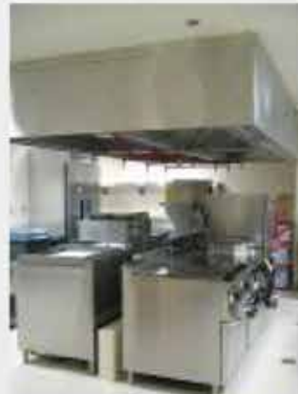
SS EXHAUST HOOD
